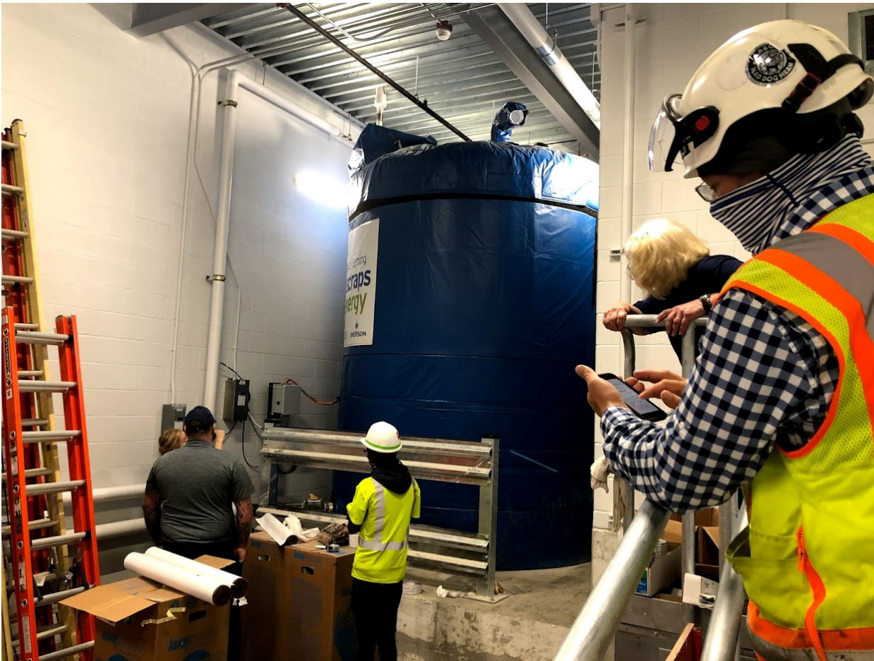
Kent State University Grind2Energy InSinkErator in the DI Hub. Kent State University photo.
