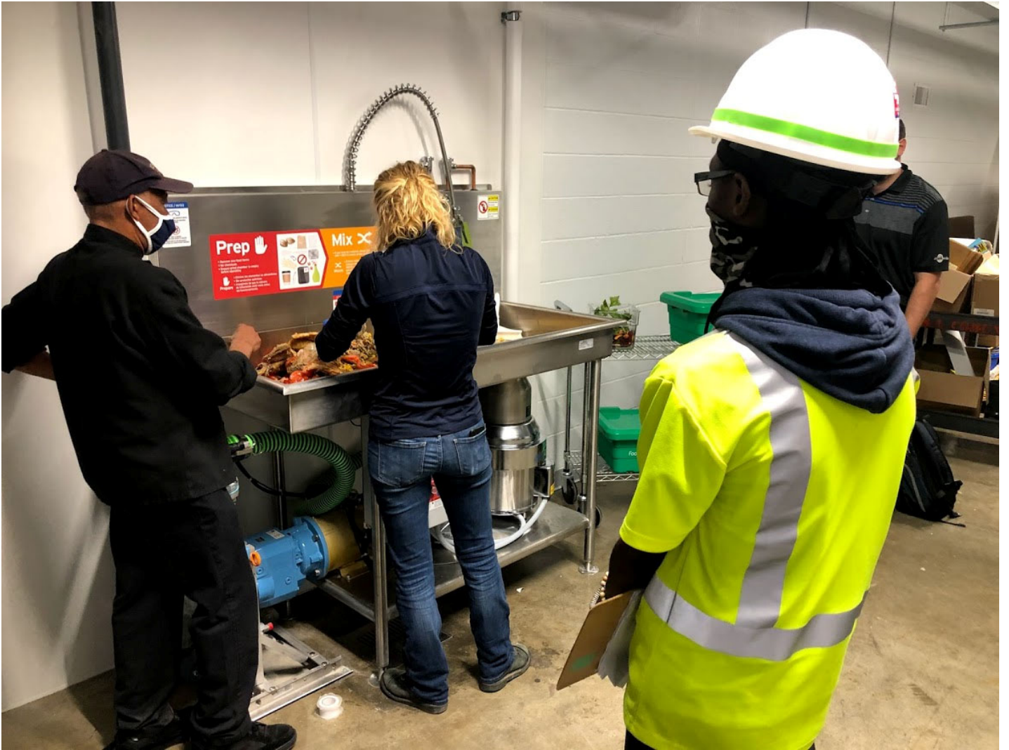
Kent State University Grind2Energy InSinkErator in the DI Hub. Kent State University photo.
